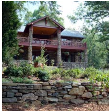
New drystone wall, meant to resemble historic stone house. Used existing, failing wall and local stone. Work of Unturned Stone.
