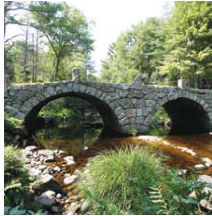
Drystone bridge built in the mid 1800's, still in use today in Hillsborough, New Hampshire. Photo by Tomas Lipps of Stonexus Magazine
