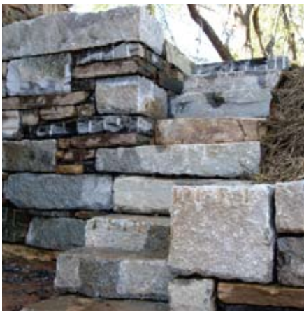
Dry stacked retaining wall and steps, granite quarry waste, reclaimed limestone, any new stone is local. My work with Unturned Stone.
